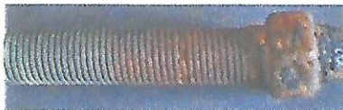
Pictures A+B: while still in place, the upper shaft and nut of the keel bolt displayed major corrosion (above). Following its removal, the extensive corrosion was further confirmed by thermal imagery (right)
